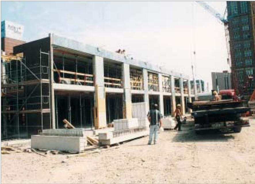
Installation of a monolithic element – façade and load-bearing structure as a single unit
